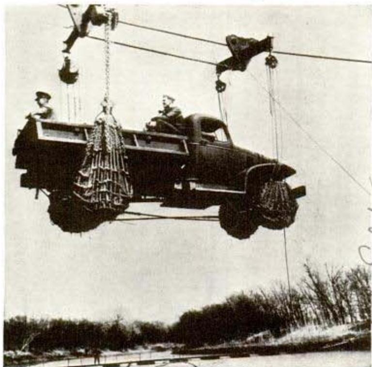
Special carriage picking up army truck and carrying it across river on cable bridge which was erected by army engineers at Fort Riley in three hours
