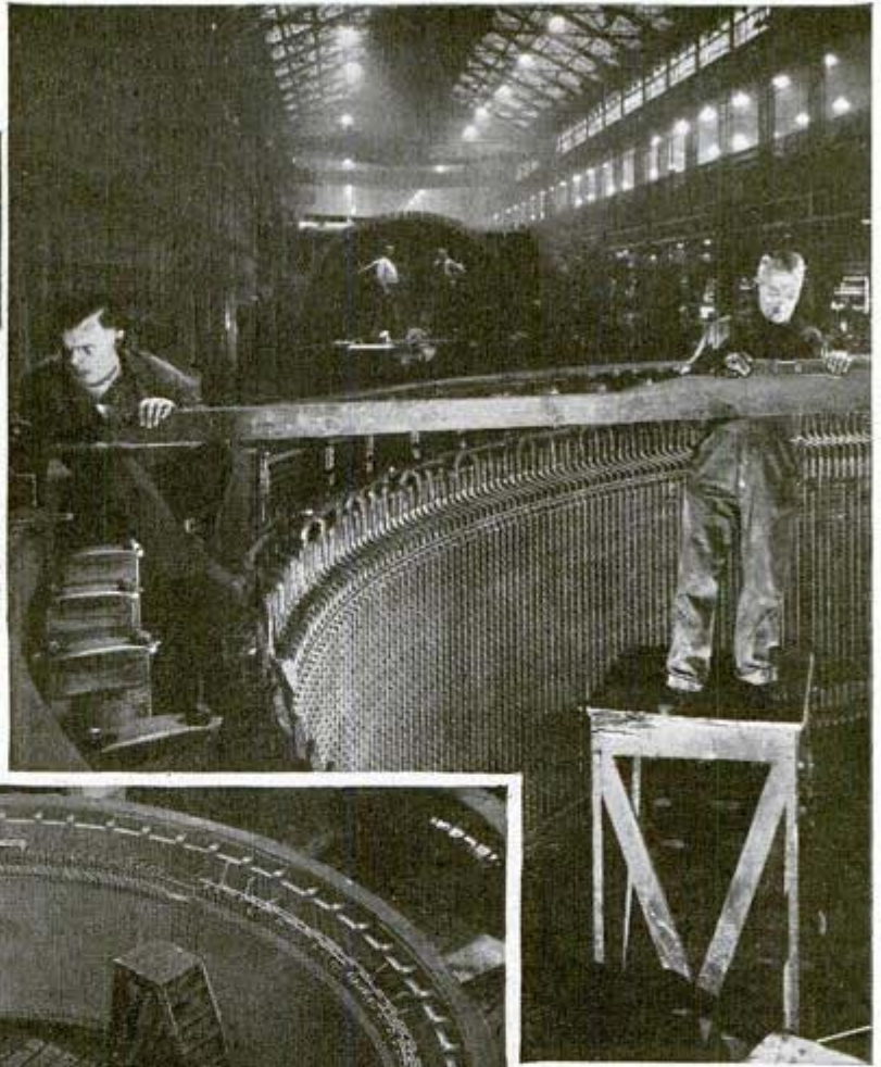
Leveling top edge of stationary member for one of the Grand Coulee waterwheel generators. This scene is in the Westinghouse works
