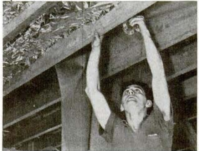
Installing tin foil above ceiling of new home to form shield against high temperatures and to prevent hot attic air from entering room below
