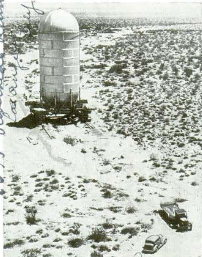
Tough orangewood logs were used as rollers as the huge tank was hauled, 300 feet a day, across a mile of rough desert
