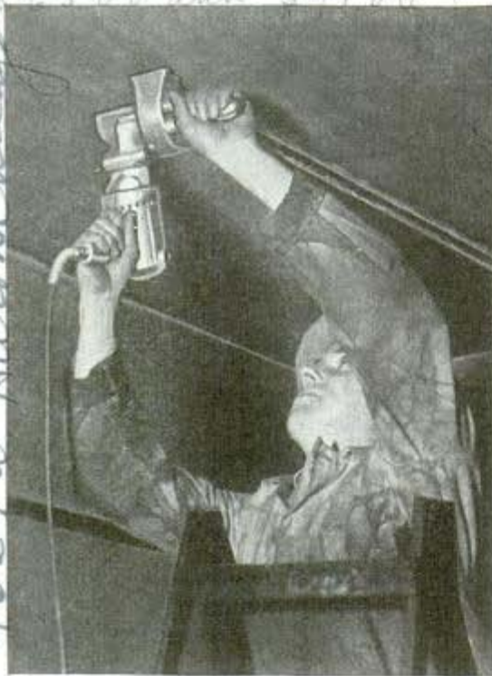
In one sweep across ceiling, twin wheels cut groove for installing electrical conduit, pipe or tubing
