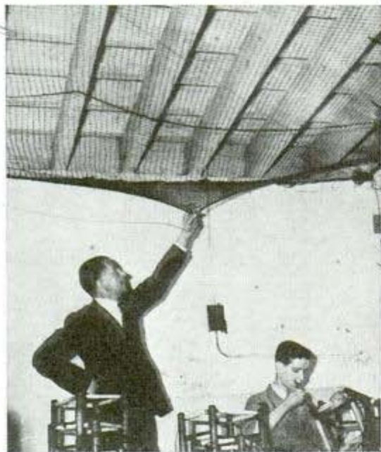
Alarm netting in ceiling of London store sounds a warning in the event building is struck by bomb
