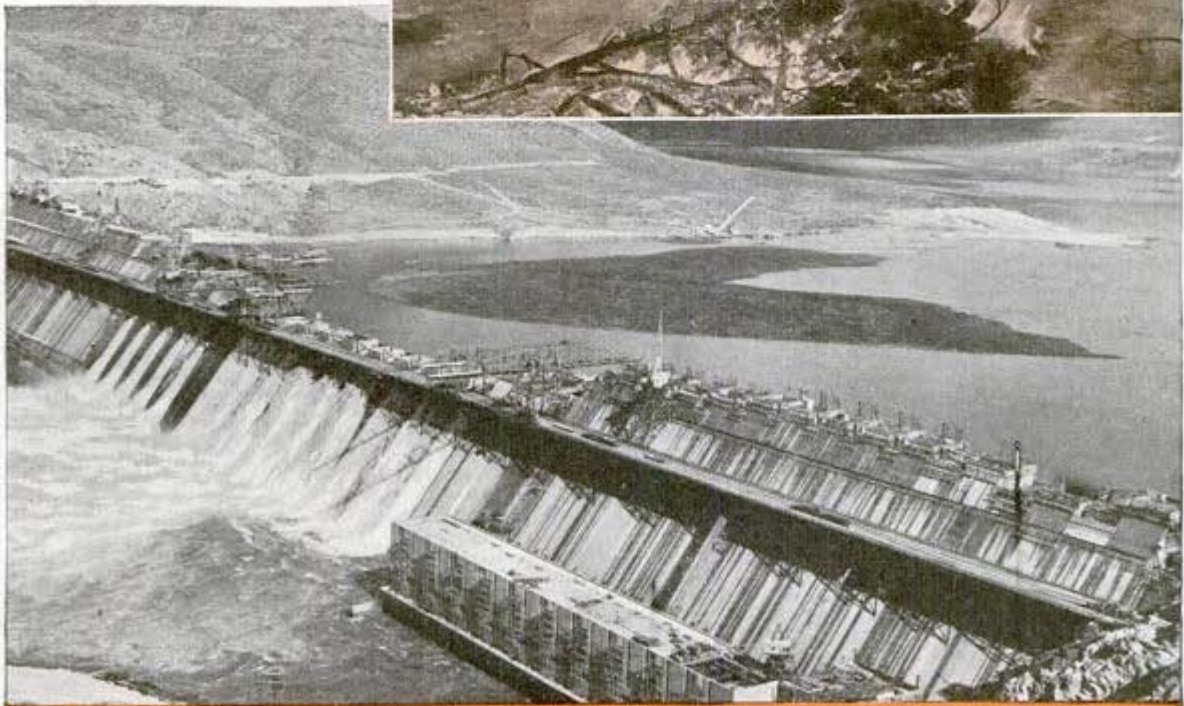
Top, clearing crew boarding barge. Center, crew at work clearing the way for Lake Columbia. Bottom, Grand Coulee dam nearing its 550-foot height. Lake will rise approximately 170 feet above level shown
