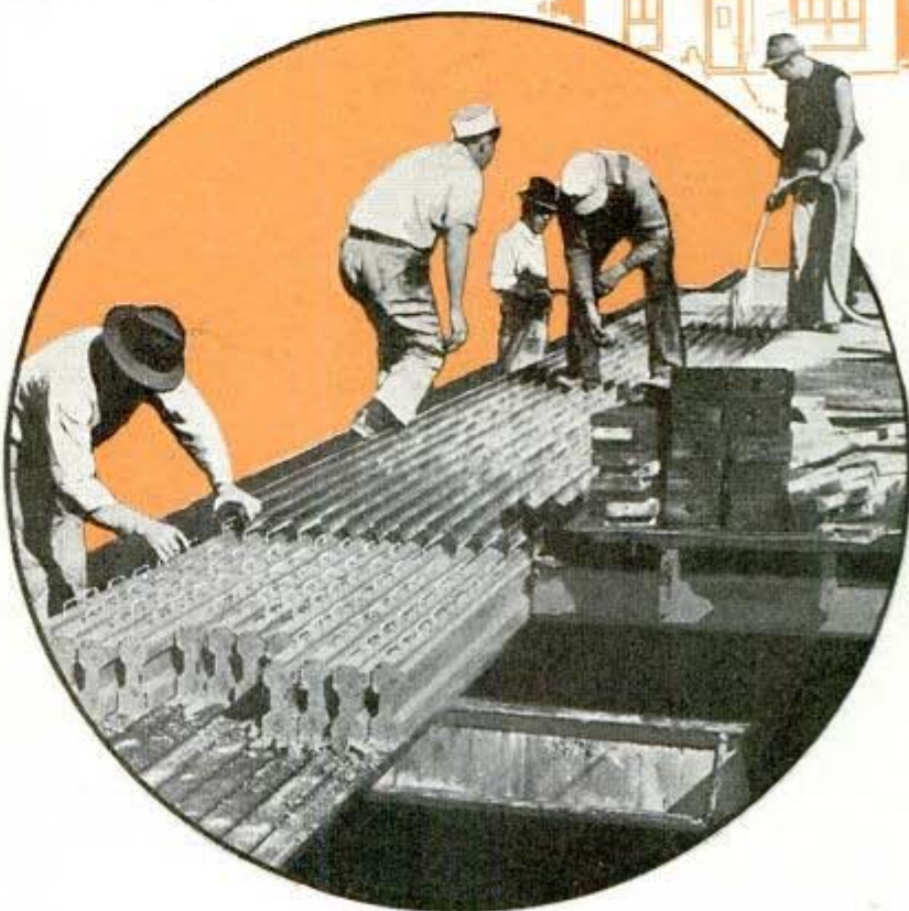
Top, concrete being hoisted from mixer to second floor. Inset, exterior of structure. Note huge beam separating floors. Circle, extruding precast joists from their forms
