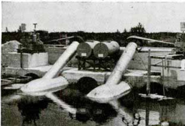
Each of these Diesel-driven pumps has a capacity of 100,000 gallons per minute
