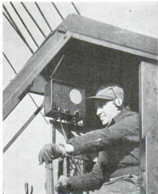
Steam shovel operator hears loud signal from headphones or loud speaker when shovel nears metal pipe
