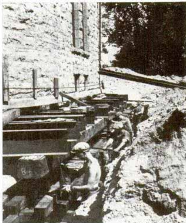
Placing jacks under 2,200-ton observatory, which was moved without disturbing delicate instruments
