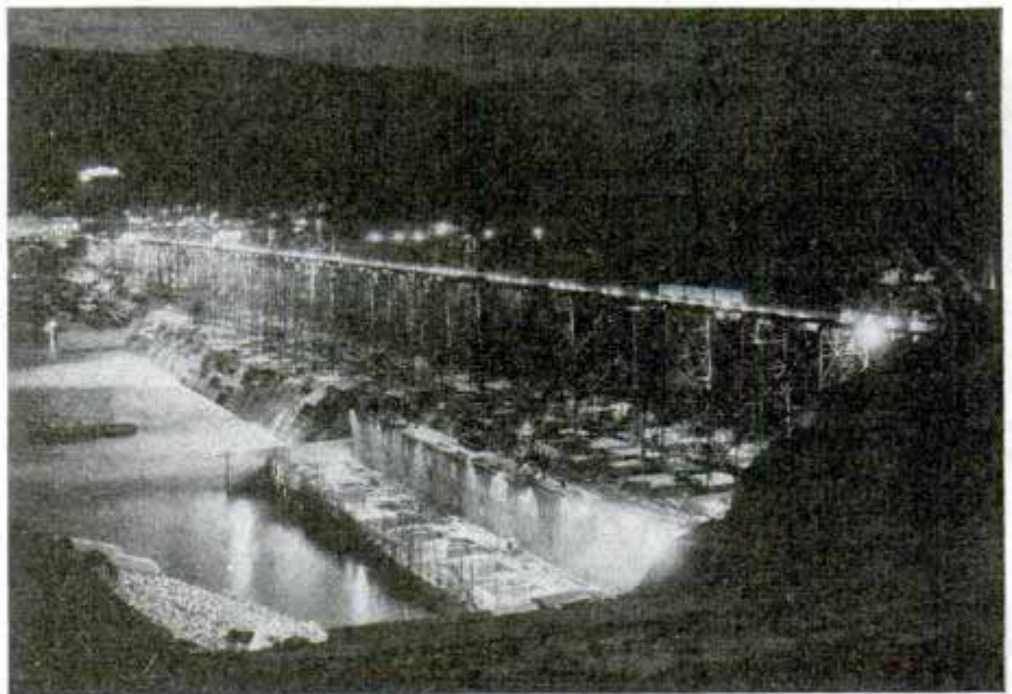
Top, left, giant concrete factory, capable of turning out enough concrete in one month to build two-lane highway more than 250 miles long. Right, watching for bedrock movements with aid of instrument combining levels, lenses and Mercoid switch. Bottom, brightly illuminated view of dam under construction at night
