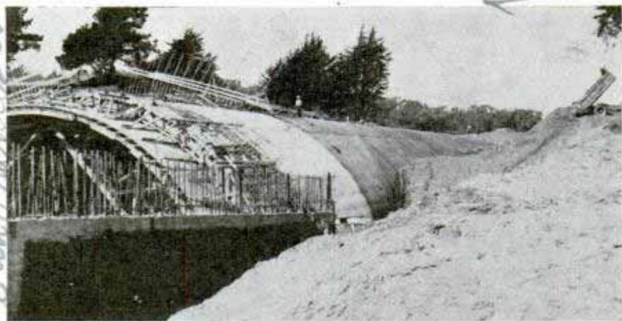
Four-lane highway tunnel traversing golf course was built in deep ditch and later covered over in order to preserve park used by army officers
