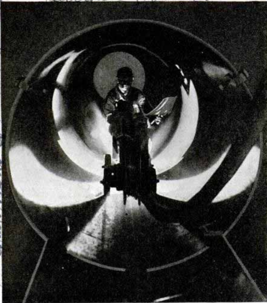
Two sheets of steel are rolled into half-cylinders, then a welder rides his machine through the tunnel and fuses halves into pipe for aqueduct
