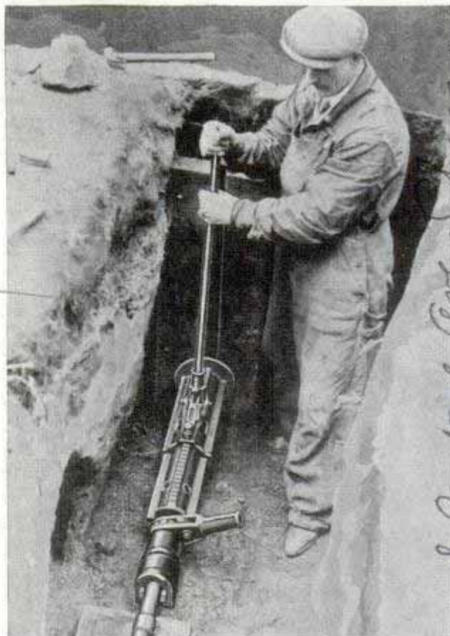
Pulling water pipe through ground with jack saves digging long ditches to reach water main in street
