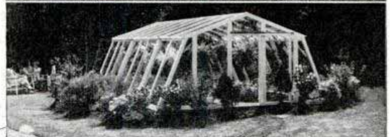
Top, right, door is added after two side sections are on foundation; center, finishing with end frame and door; bottom, greenhouse completed
