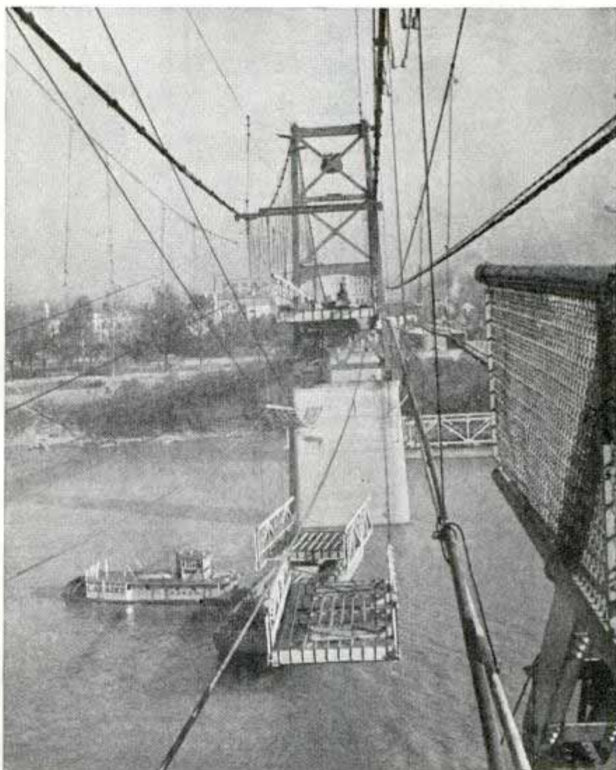
Lowering one of five sections of center span to barge in river to relieve weakened cables of their weight so they may be replaced with new ones
