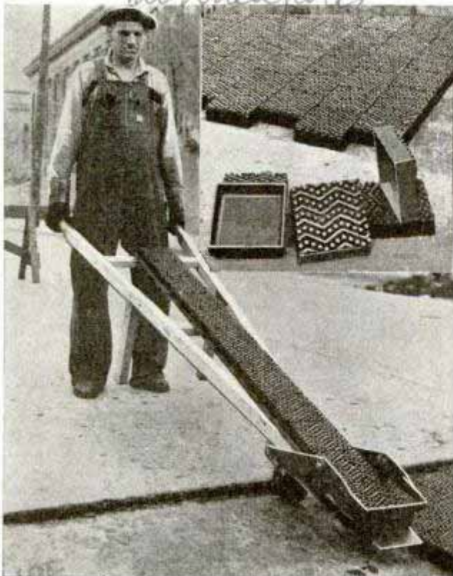
Laying cast-iron blocks in section of highway. Inset shows close-up view of their construction
