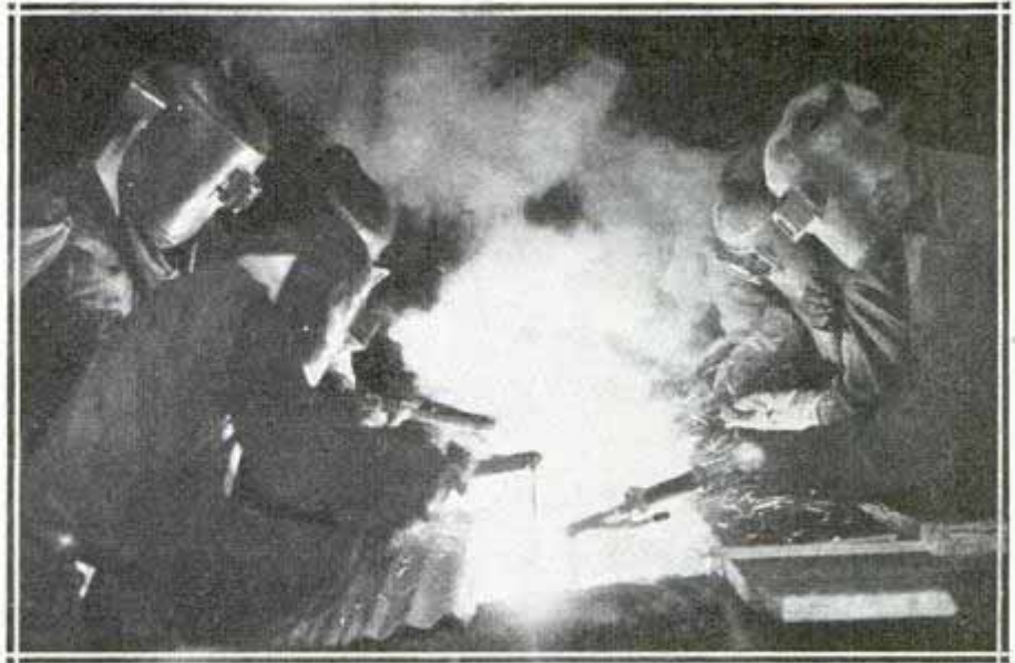
Working like a team of surgeons over a hospital operating table, six electric-arc welders melt 400 pounds of electrodes in repairing a casting
