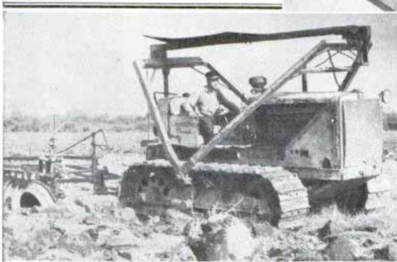
Right, tractor with sharp-nosed ram held aloft clears small brush off land with heavy blade. The tractor is Diesel-powered
