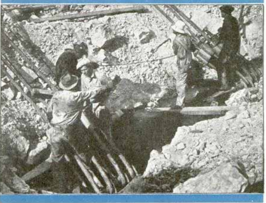
Top, right, riggers at work on one of the piers for railroad bridge downstream from Shasta Dam. Bottom, tightening cable jewels in east anchorage of new bridge
