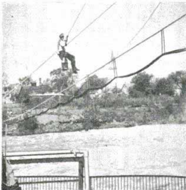
Putting a cable across a raging torrent after the bridge had been swept away by high water
