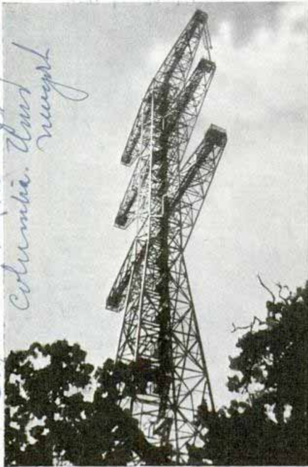
Giant tower of new ultra-high frequency station. Note the 150-foot crossarms
