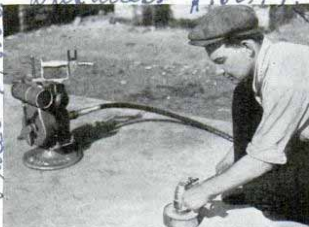
Finishing a concrete surface with hand tool driven by a portable gasoline engine
