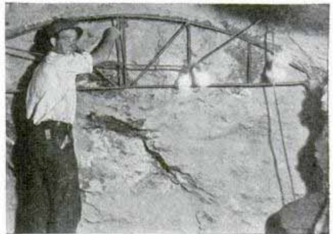
Engineer marking contour of tunnel as guide to drillers in preparing blast holes
