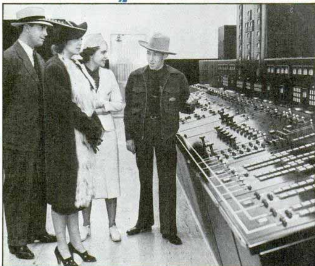
One of the switchboards in the control room at Boulder dam from which the flow of power is regulated
