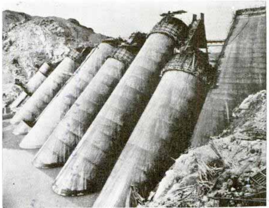
Nearing completion, Bartlett dam will be the highest multiple-arch dam in the world, storing 200,000 acre-feet of water for irrigation
