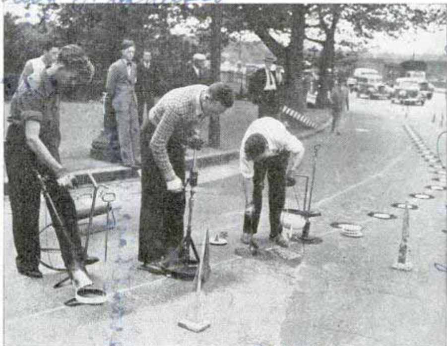
Photo shows successive stages of heating asphalt, preparing recess, lining it with hot tar and then laying non-skid traffic markers in place
