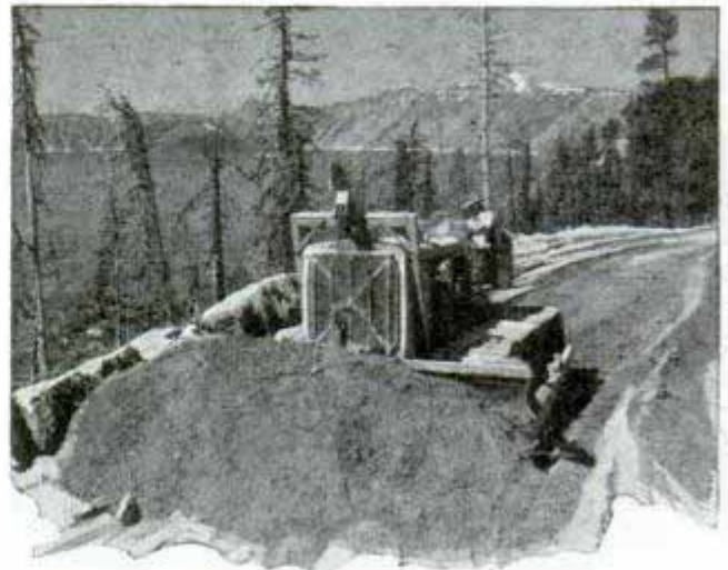
Tractor equipped with bulldozer building rim road at east edge of Crater lake
