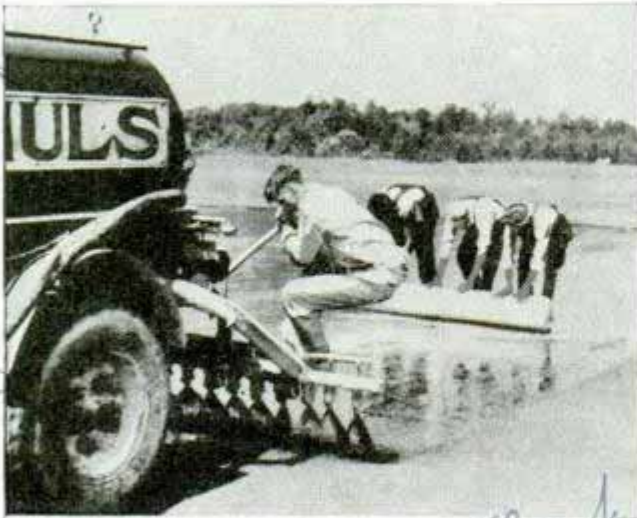
Three men unroll cotton binder on airport runway after truck lays down adhesive coating of tar
