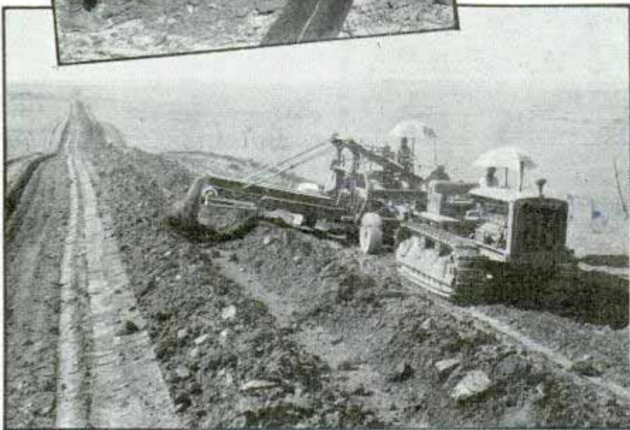
Top, one man does work of many with this tractor-scraper combination. Center, earth-borer digs hole and sets in pole. Bottom, elevating grader building mile in fifteen hours moves 6,000 yards of earth per mile
