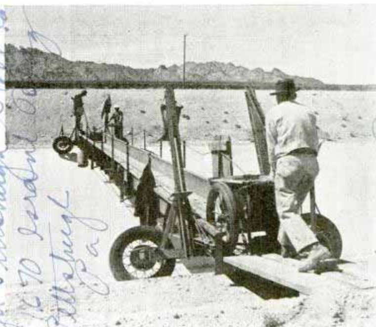
Rolling cement across bridge that moves along the canal on wheels at either end
