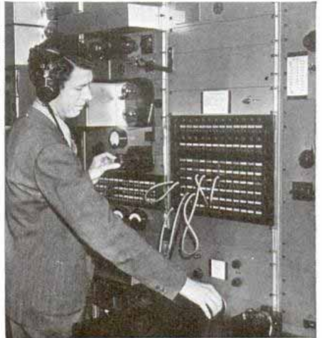
Switchboard in sound laboratory through which sounds from different stages are switched to proper recording machines
