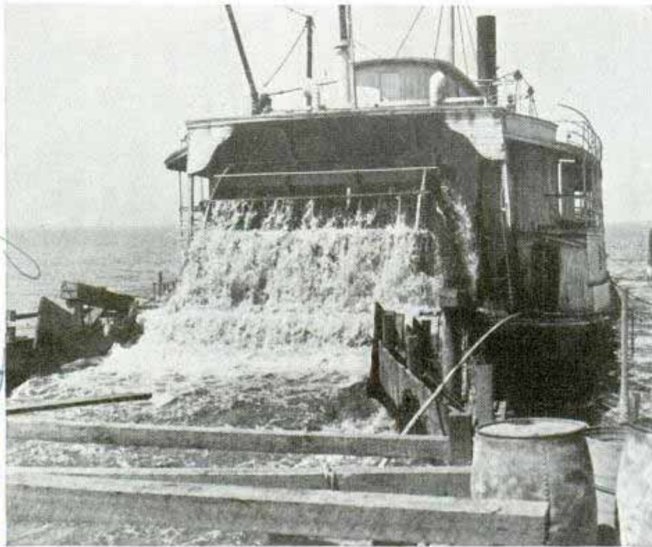
Old steamer at work pumping floodwaters out of island. The water is pumped up over the levee and down into the river
