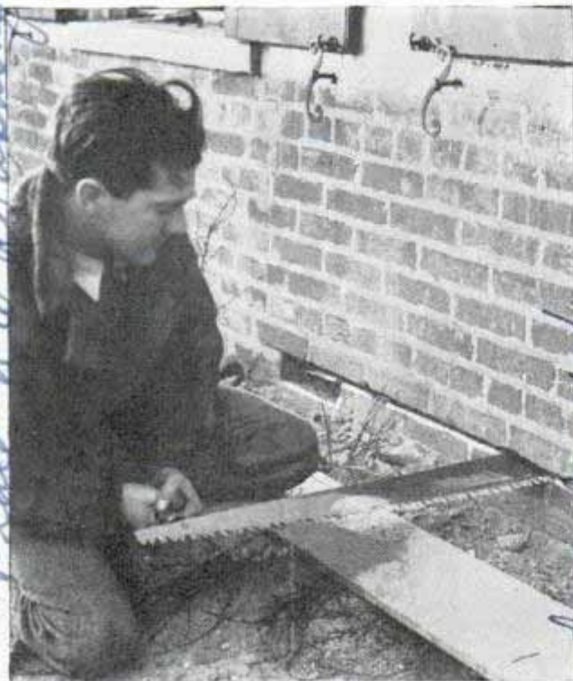
After sawing out one layer of mortar with crosscut saw, copper sheet is inserted for insulation
