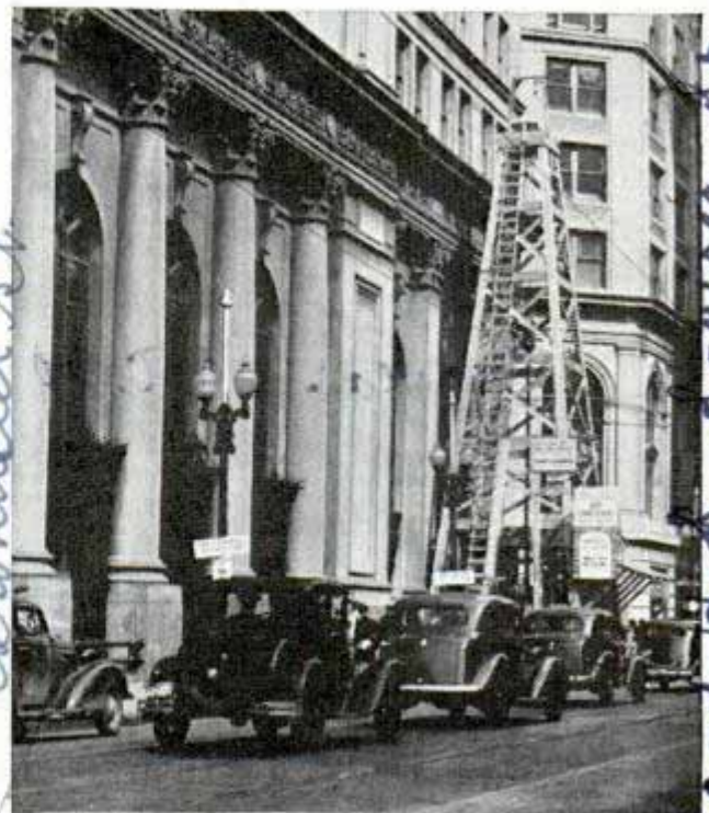
Here is a derrick set up in a busy city street to drill for water
