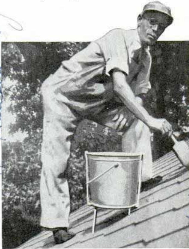
Working on a gable roof, the painter adjusts the legs of bucket holder to keep the can level
