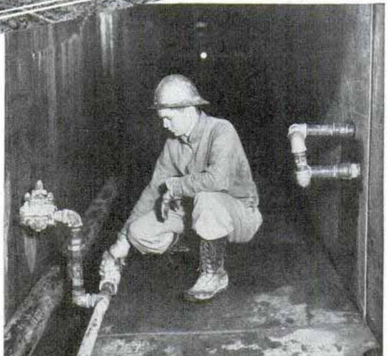
Top, taking temperature readings of concrete mass. Center, strain meters which are buried in concrete. Bottom, header pipes for cooling system extend into galleries of dam
