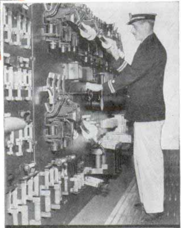
Top, throwing switches that turn off radio transmitter, and actuate loop direction finder. Bottom, main electrical switchboard of ship from which current is supplied for operating radio, lights, pumps, and other equipment
