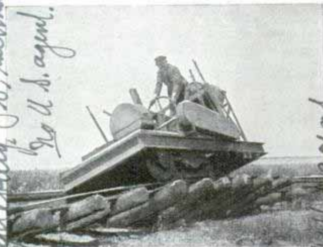
Track shifter being used to move rails and cross-ties into a new position
