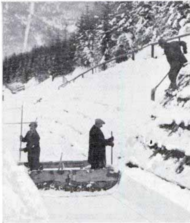
Another step in the construction of the run, which is carefully engineered
