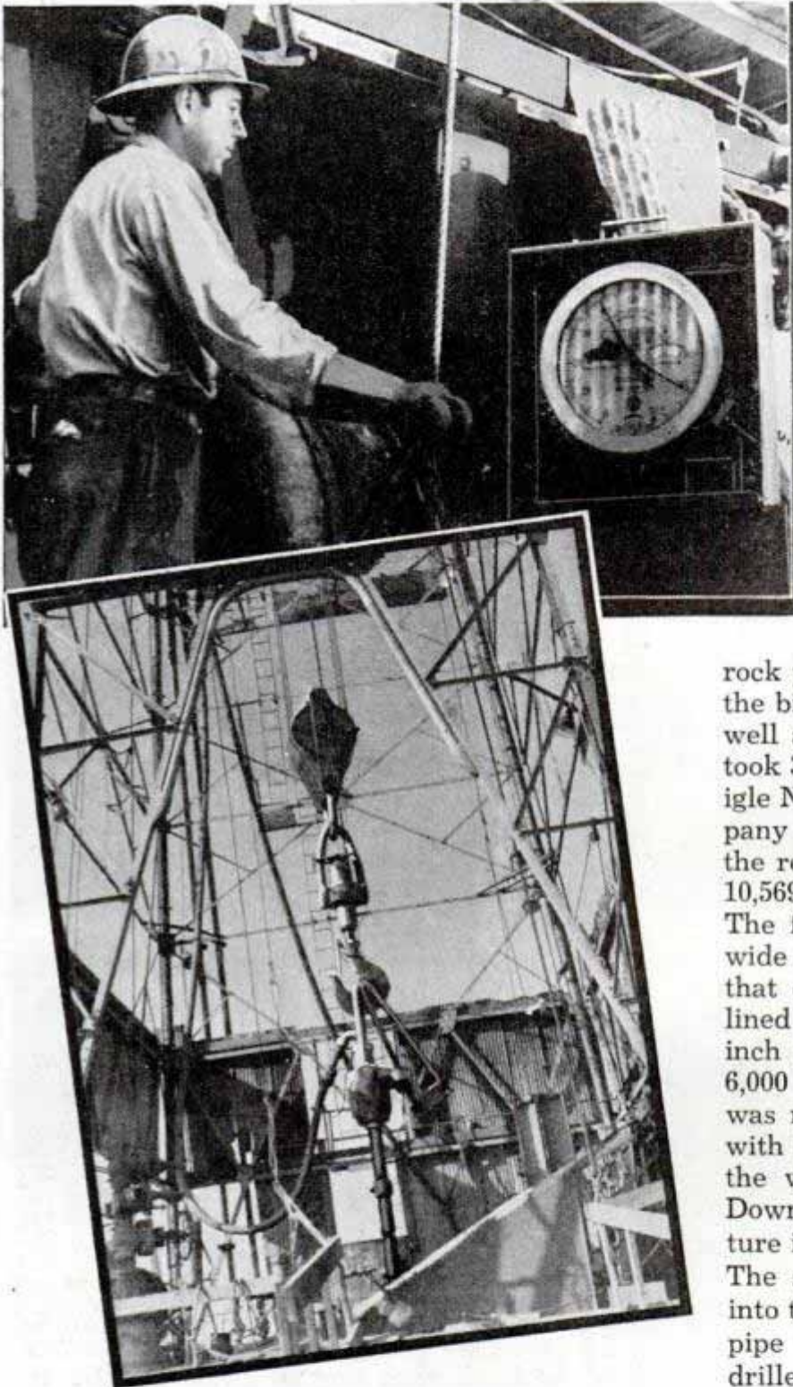
Top, driller at the controls. Bottom, derrick floor, showing traveling block and swivels that support part of drill pipe's weight
