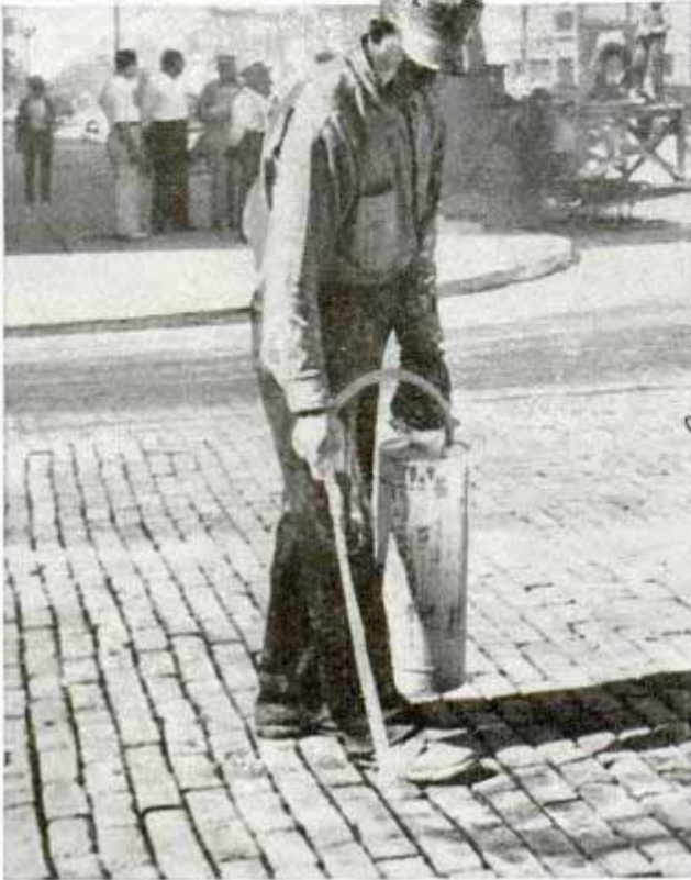
Whitewashing bricks before tarring crevices makes it easier to remove excess tar from surface
