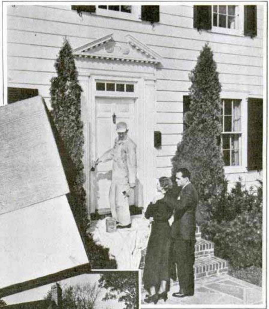
Right, painting house with self-cleaning white. Center, comparing ordinary white paint with self-cleaning type after weathering. Note how much whiter is the self-cleaning paint, shown below. In bottom photo, house remains white after long periods of weathering
