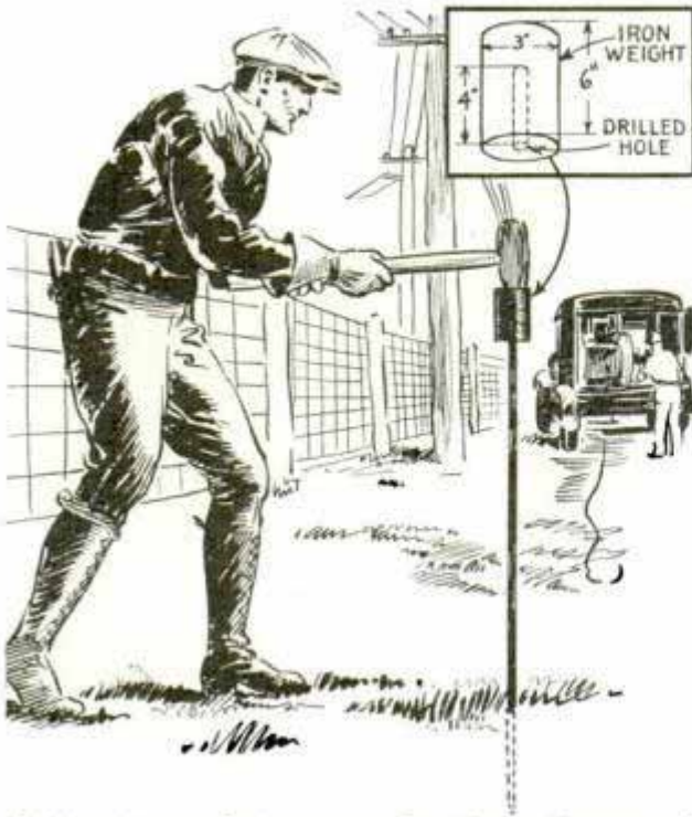
Driving iron rods into ground with weight on ends prevents vibration which causes buckling
