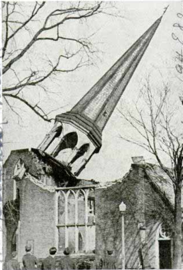
Hundred-foot steeple toppling into ruins of church as tractor pulls down supporting columns
