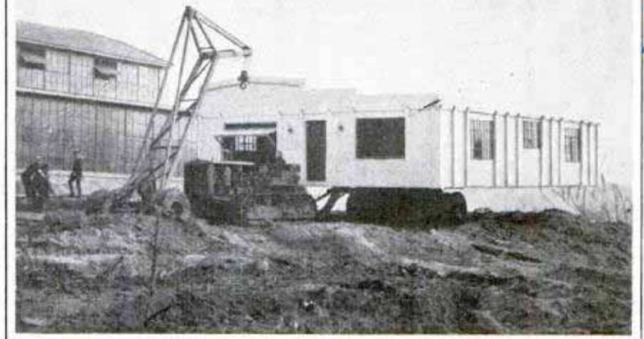
Five-room welded steel home being completed in factory and moved to site, where a crane lifted it from sixteen-wheel trailer and set it down
