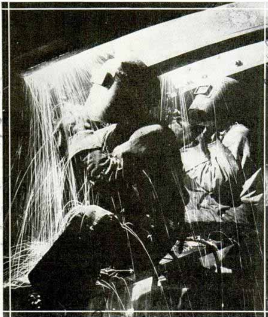
This spectacular photograph shows two welders at work in tunnel. Note (in foreground) the white streaks produced by flying sparks
