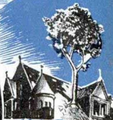
TREE GROWING ON ROOF
