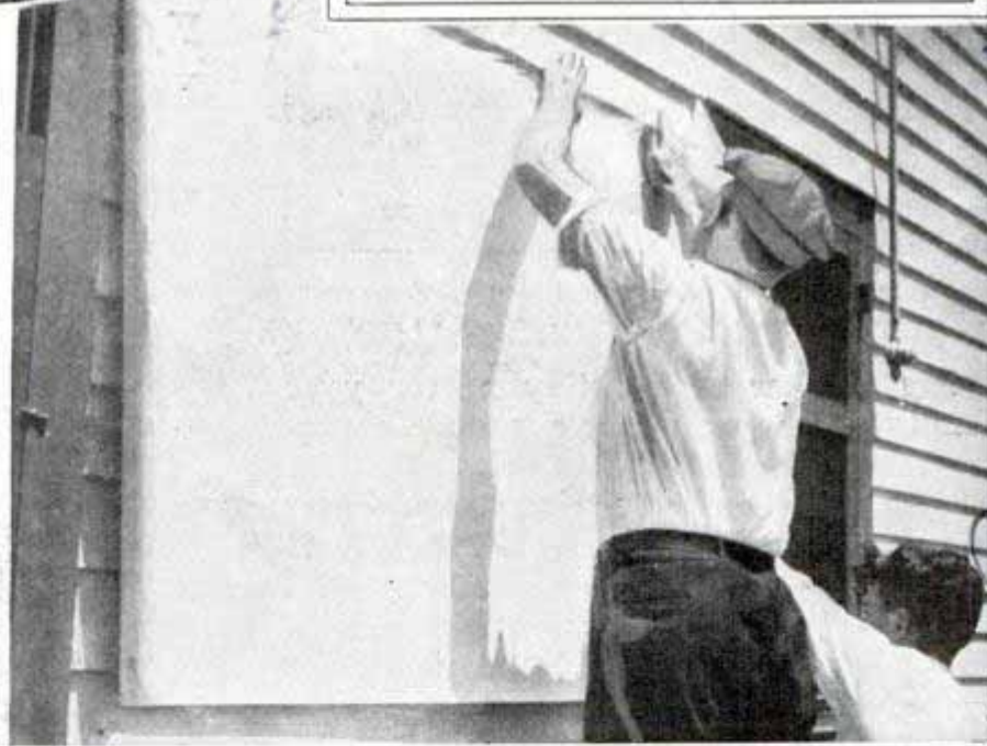
Top, left, brushing on cement. Bottom, applying the cloth-backed paint. Top, right, trimming to fit at ends of the boards
