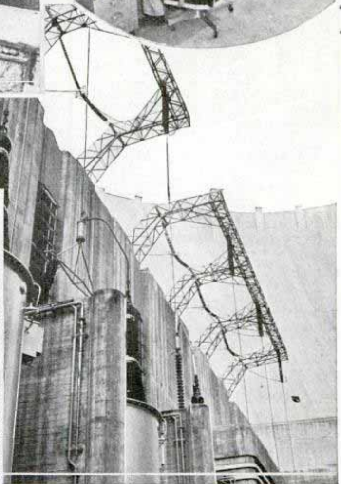
Top, left, observation point with Lake Mead, now 385 feet deep, below. Right, automatic telephone switchboard and powerhouse control board. Bottom, left, looking from exciter platform atop 115,000-horsepower generator. Right, transformers on face of dam handle the flow of power from the big power project through substations to Los Angeles, Calif., 266 miles away
