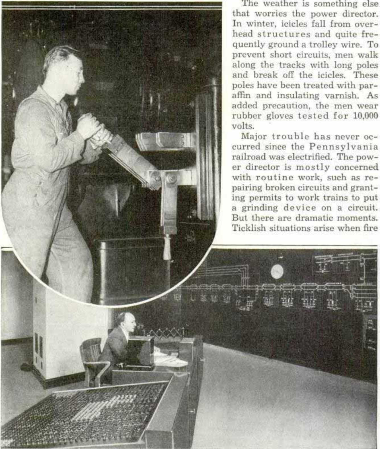
Load dispatcher's office in the Pennsylvania station, Philadelphia, and, above, throwing a switch in a power sub-station
