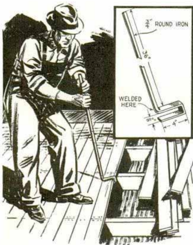
This simple tool solves the problem of removing old flooring for the inexperienced workman
