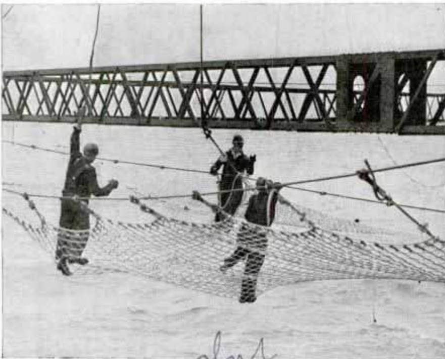
Testing life net which has been spread beneath giant Golden Gate bridge to prevent workers from falling into water
