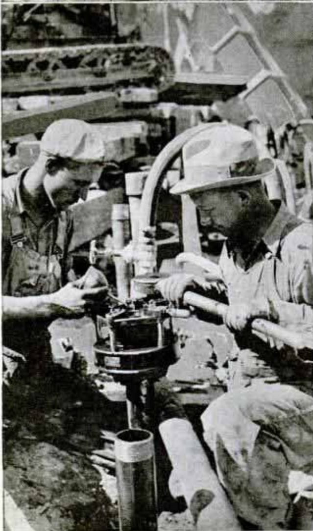
Brine circulated through deep-driven pipes freezes soil and checks landslide of clay mountain at brink of excavation for dam. Below, threading a pipe
