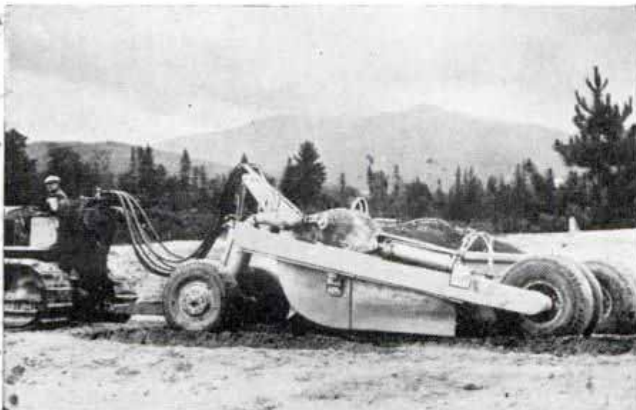
Road-working robot in action. Note hydraulic hose connections to tractor, permitting driver to apply power where needed in the machine
