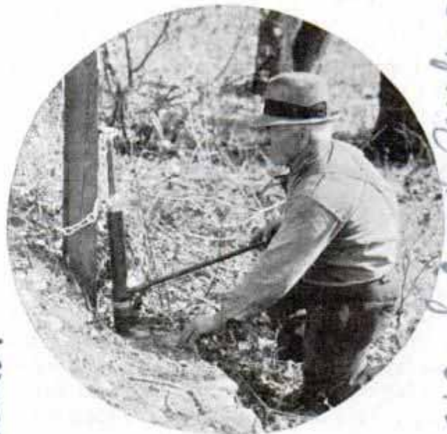
Jerking a fence post out of the ground is a simple job with a hydraulic auto jack and chain
