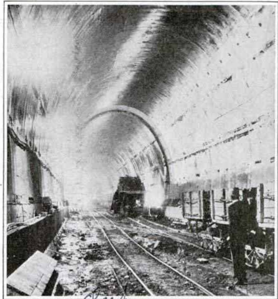
This photo gives you an idea of the size of the big water tunnel which will serve San Francisco. It is being rushed to completion
