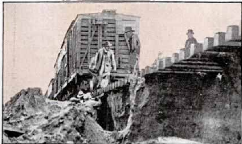
Clearing flood debris from telephone poles so switchboard, center, can function. Bottom, repairing railway trestle which was undermined by flood waters
