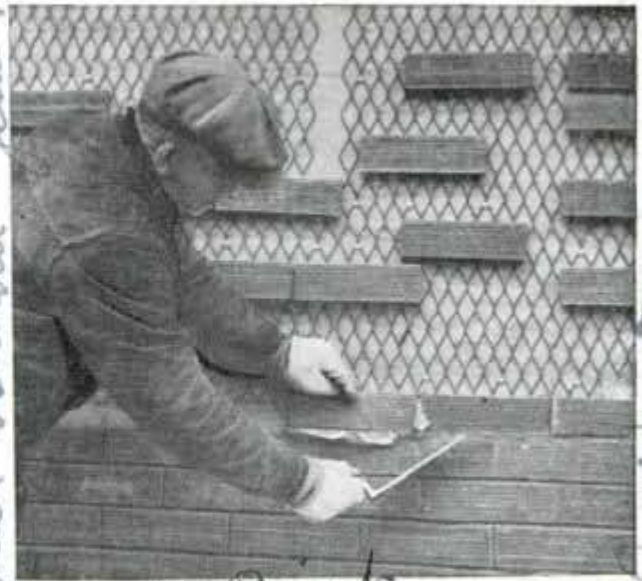
Thin bricks are properly aligned and supported by prongs on mesh nailed to old wall of house
