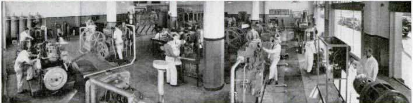
Partial view of Diesel-engine operating room— one of the important Departments at National Schools.
