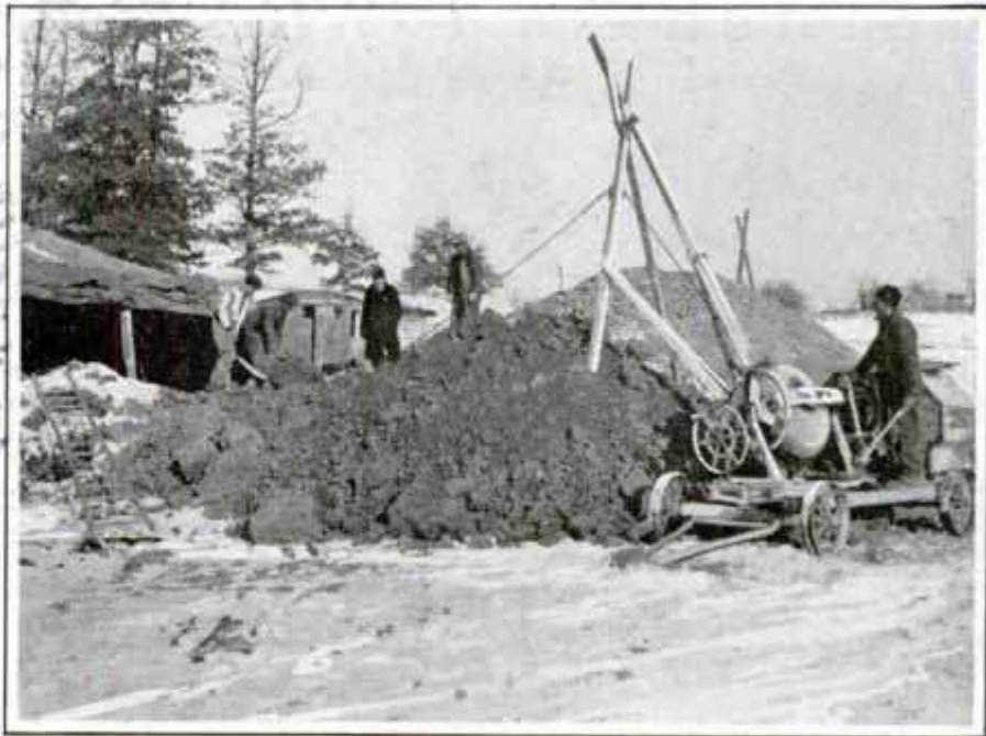
Removing dirt from house excavation. Note tent at left which protected workers from cold on this winter building job
