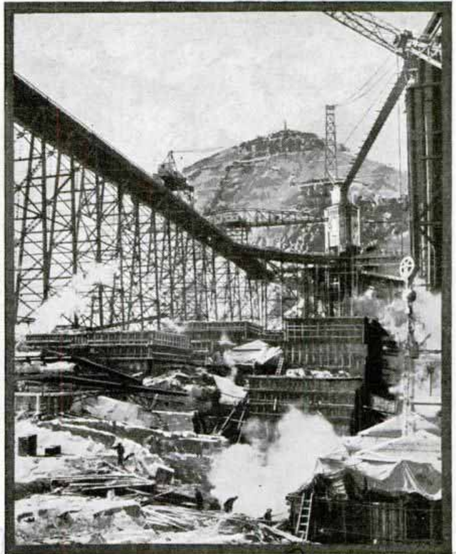
Steam Shooting live steam under the canvas "blanket" keeps new-poured concrete of the Grand Coulee dam from freezing before it has set properly
