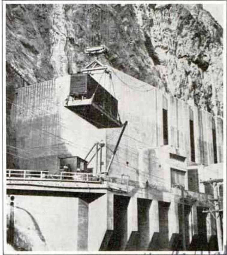
Loaded freight car swings out over canyon on cableway and drops 800 feet to rails leading to Boulder Dam power plant
