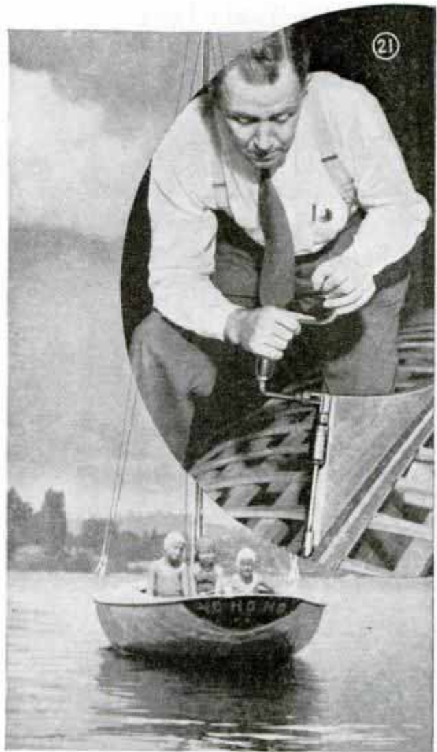
About the last thing you do before planking is to bore the hole for the rudder post as in Fig. 21. The after end of the skeg is used as a guide
