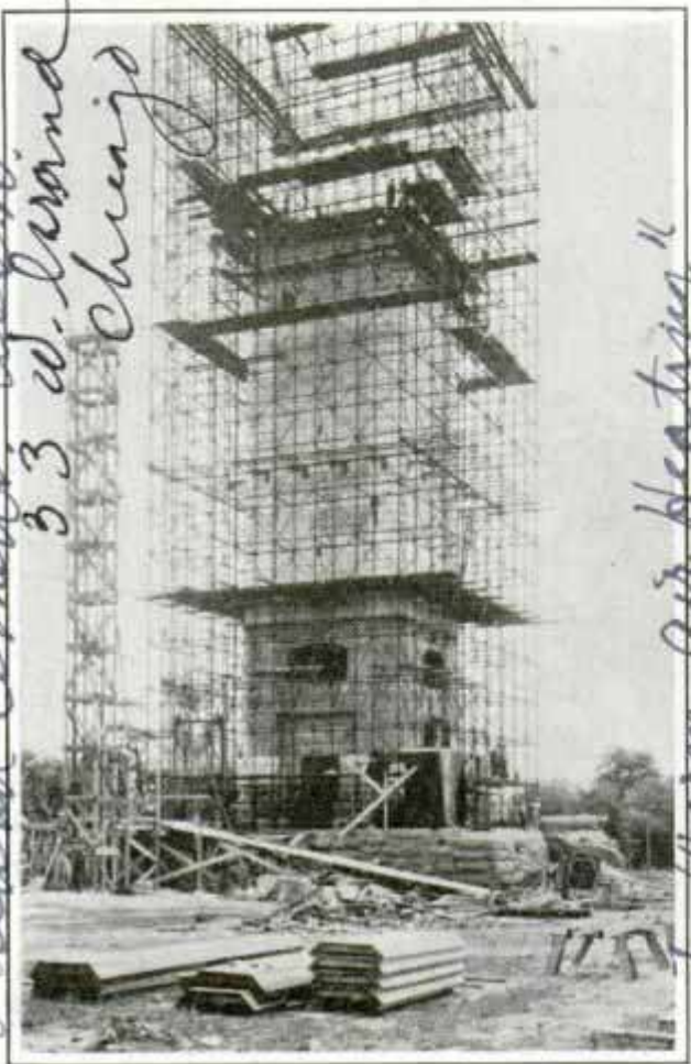
Concrete tower being constructed by method that cuts costs and speeds up the work
