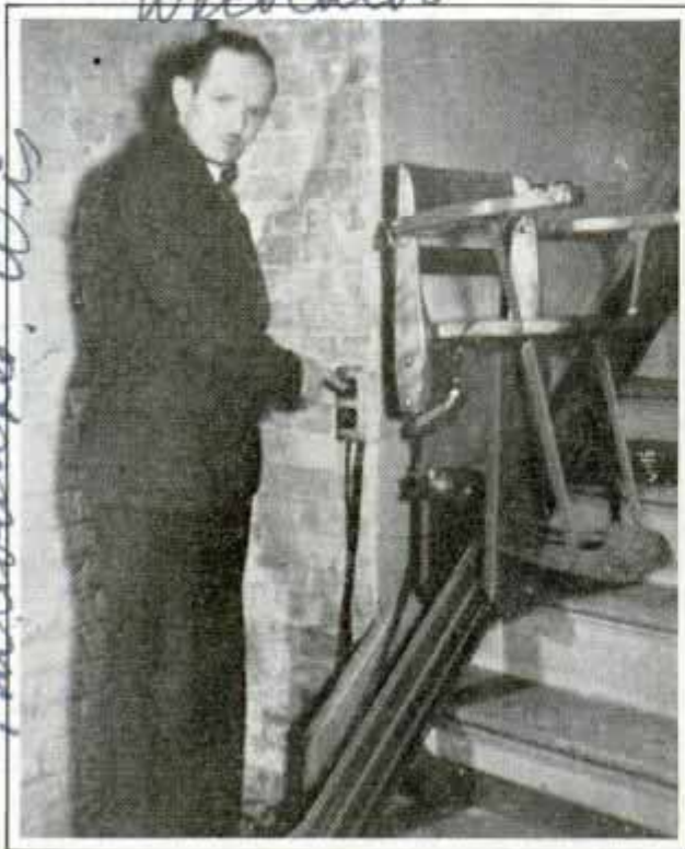
Operating switch on elevator which is installed on stairs without marring woodwork
