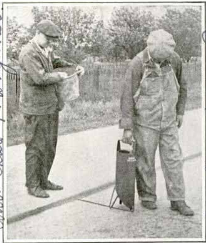
Applying Asphalt to Crack between Concrete; Note Ease of Using New Container
