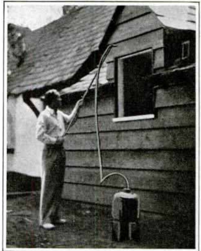
Gas Torch Used for Burning Exterior of Cabin to Antique It and Preserve the Wood
