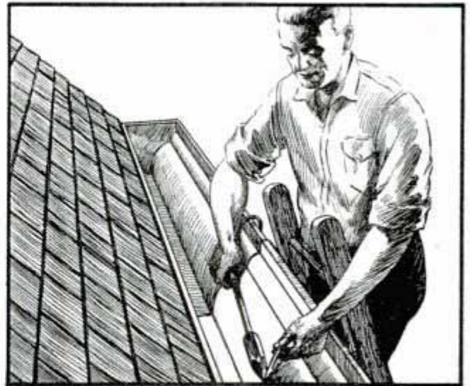
Leaky Eave Troughs Repaired by Soldering New Pieces of Trough over Damaged Portions
