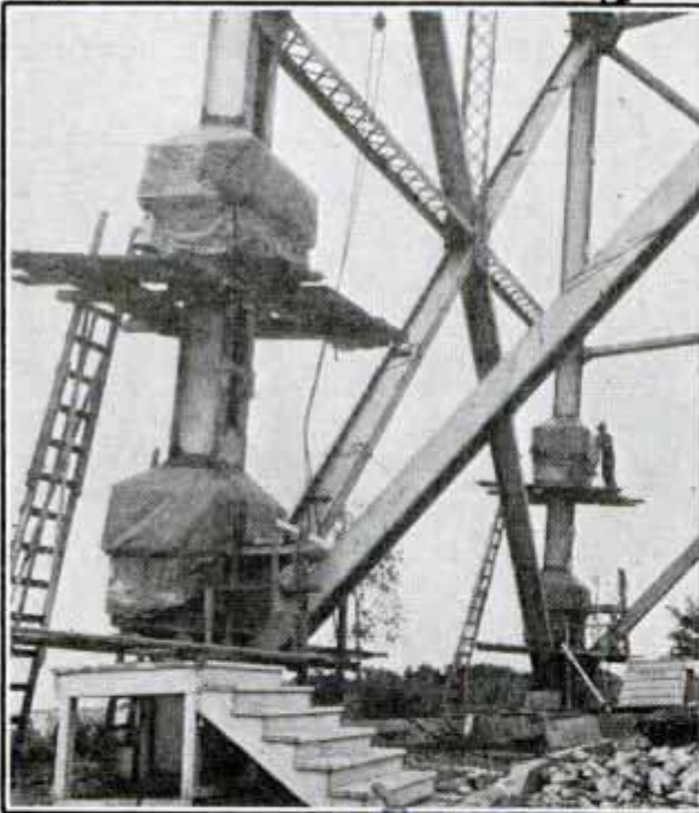
East Tower of Skyride Crashing after Two Legs Had Been Melted by Thermite in Cupolas, Below
