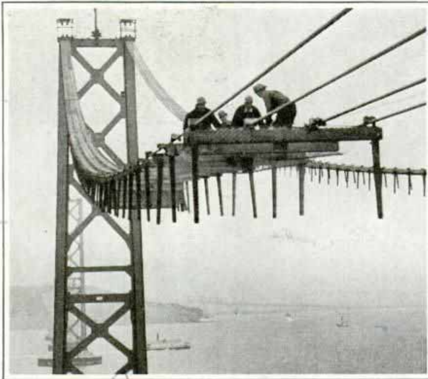
Daring Workers Are Shown Stretching Narrow Catwalk That Will Be Used in Stringing Cables to Support Big Bay Bridge
