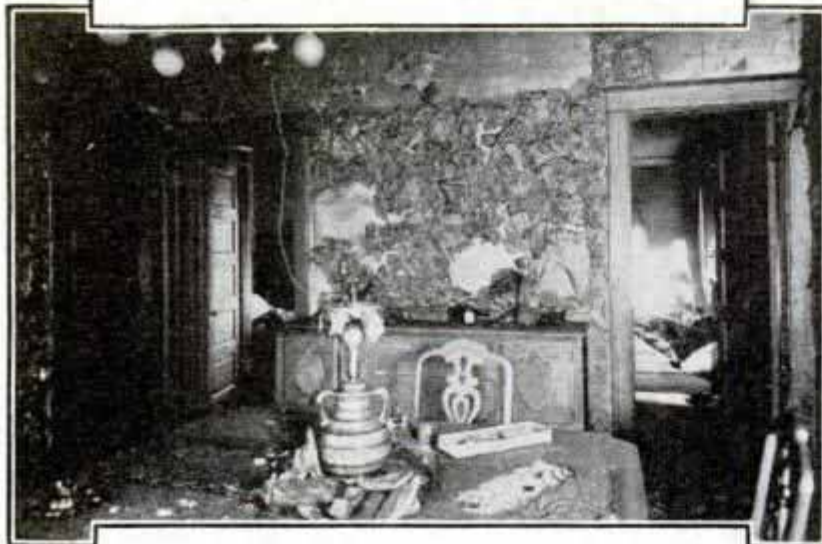
Note the Evenly Burned Walls Indicating They Had Been Sprayed with Some Combustible Liquid; the Man Who Started the Fire Confessed after This Picture Was Presented
