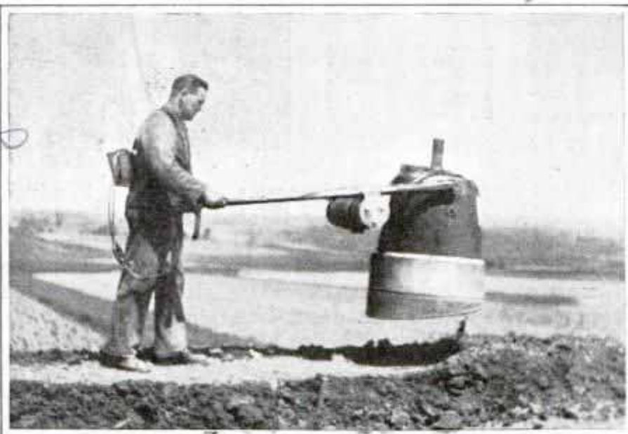
Operating the Jumping Road Tamping Machine; Internal Explosions Force the Heavy Tamper into the Air, as Shown in Photo
