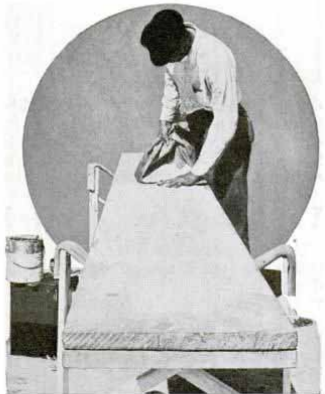
Liberal Coatings of Paint and Sand Give Diving Board Nonslip Surface to Prevent Accidents
