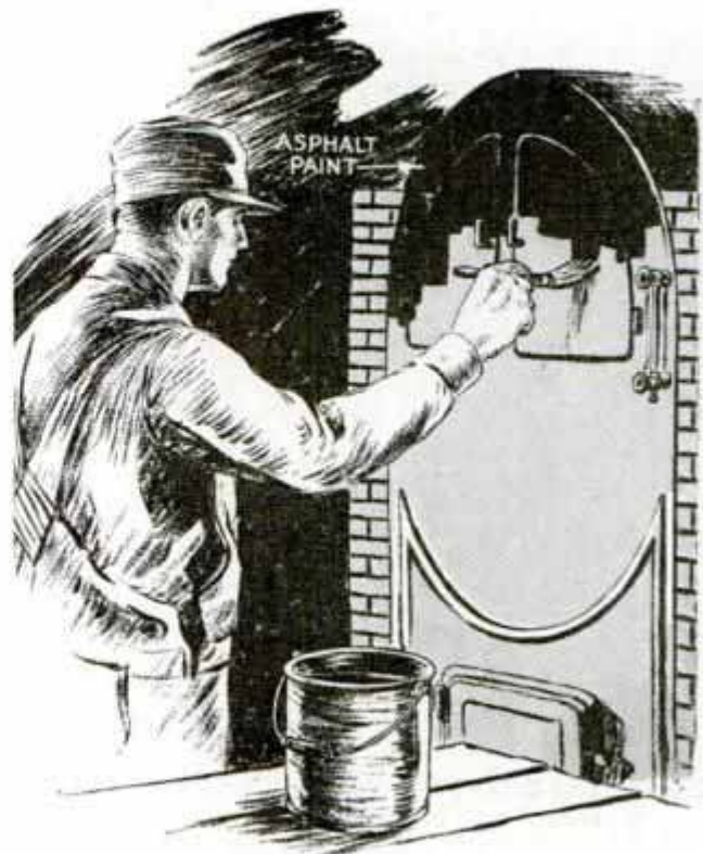
Paint Mixed with Common Asphalt as a Base Is Not Affected by Heat from Boilers
