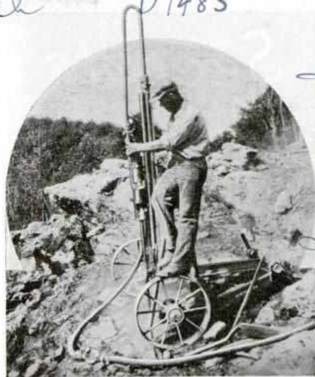
Wheeled Carriage Supports Rock Drill in All Positions So One-Man Operation Is Possible
