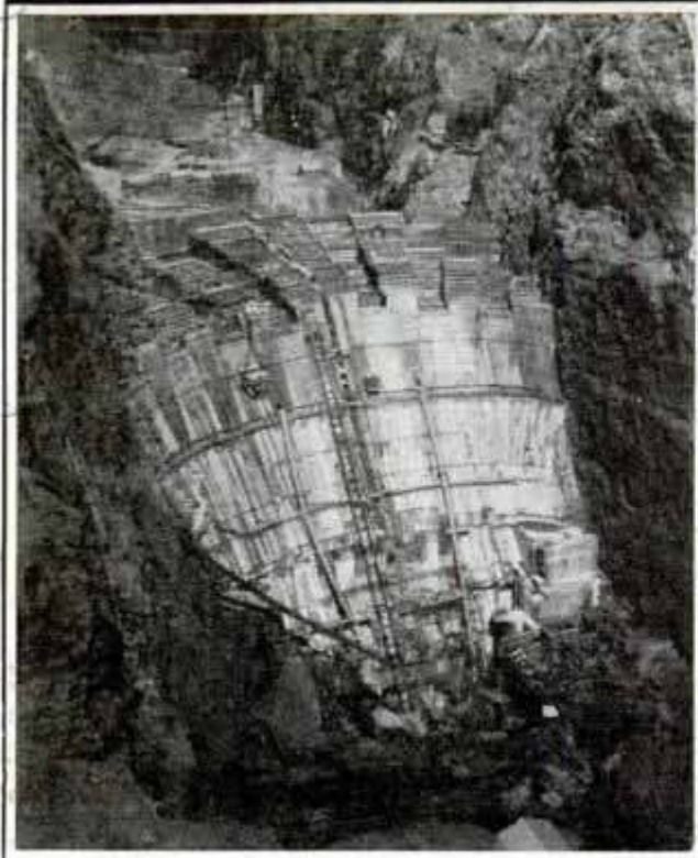
Above, Plan for the Bonneville Dam in Oregon; Below, Boulder Dam When About Half Finished
