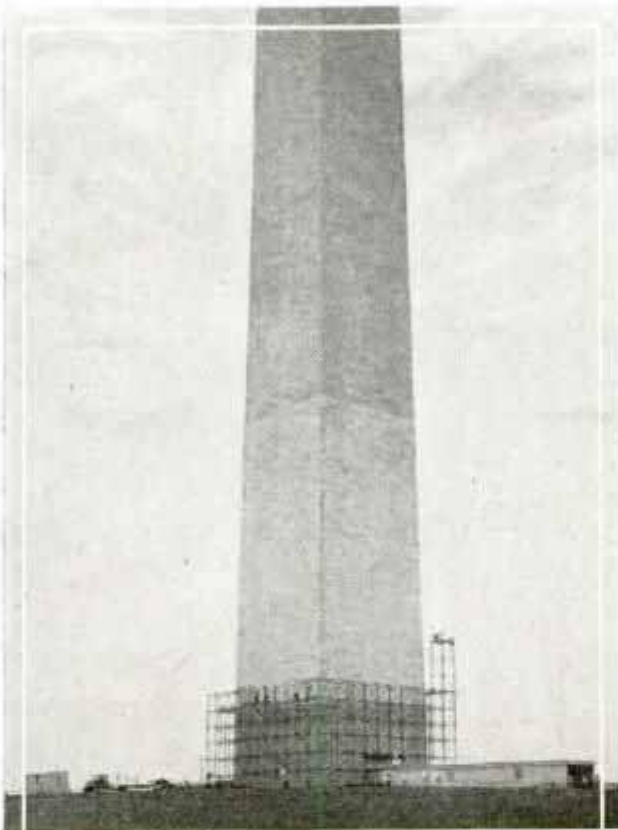
D/1102 Metal Scaffold around Washington Monument from Which Workmen Are Repairing the 555-Foot Shaft
