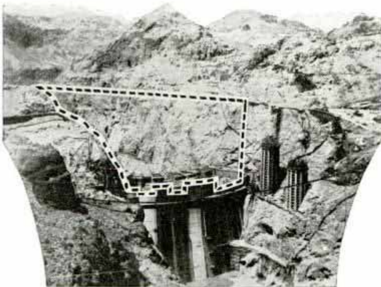
© International News Photo Dotted Line Shows Work Yet to Be Done on Boulder Dam, While Below Is the Completed Section
