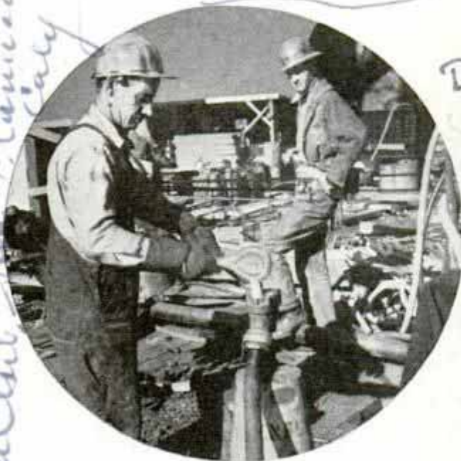
Dropping Hot Rivets in Pneumatic Metal Tube to Be Carried Up to Bridge Workers
