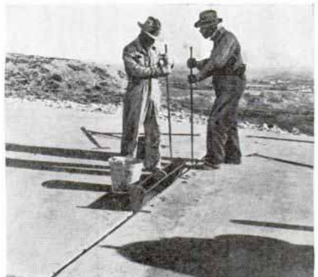
Cotton-Seed Hulls Mixed with Asphalt Used to Fill Expansion Joints in Concrete Roads
