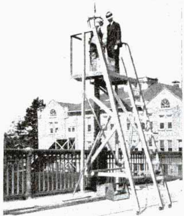
Platform Used as Safety Measure in Hanging Fixtures on Lamp-Posts of High Suspension Bridge
