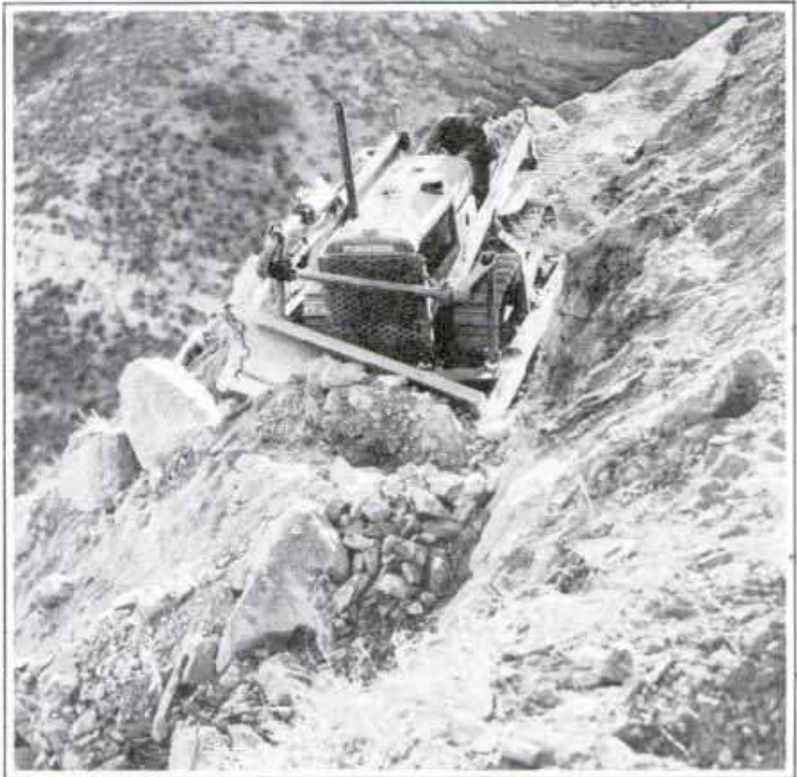
Adjustable Bulldozer Run by a Tractor Which Builds Mountain Road by Digging Off the Upper Side and Filling in the Lower Side
