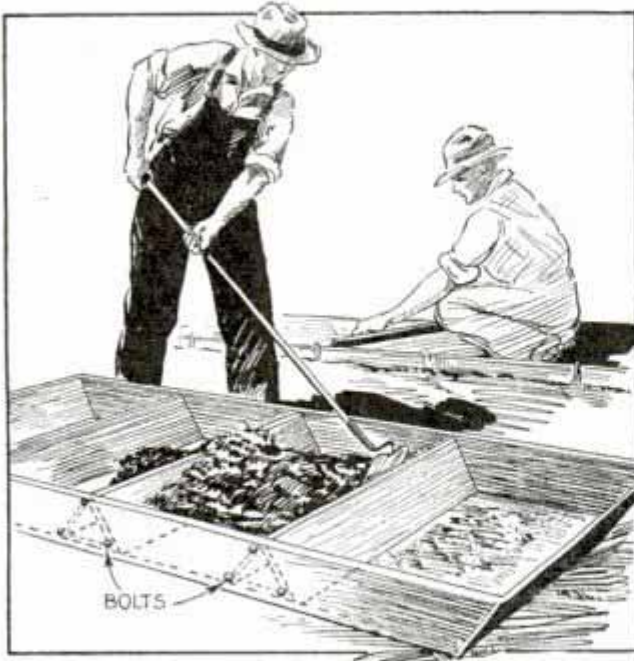
Slanting Partitions Bolted to Sides of Mortar Box Save Labor in Mixing Concrete
