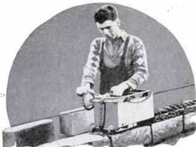
Mortar Spreader Operated by Turning a Crank; It Does the Work of Three Men
