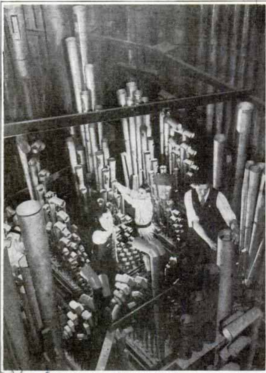
Installing Some of the 10,491 Pipes in a Big Organ; This Instrument Contains 176 Draw Stops and There Are Four Keyboards
