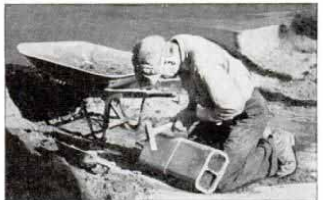
Tile Parted by Packing It with Wet Sand and Then Tapping It Lightly with Hammer
