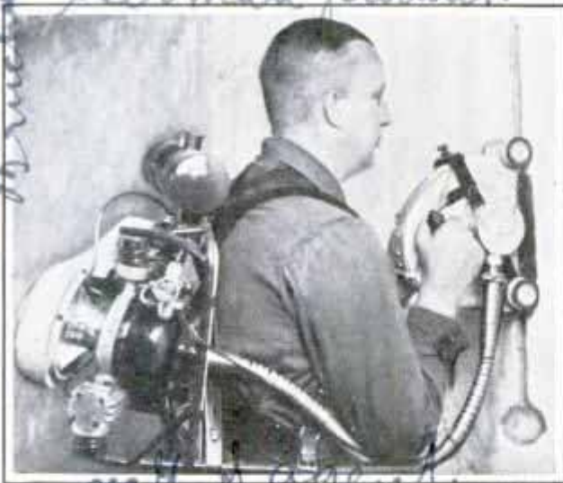
Cutting Groove in Wall for Electric Cable; Note Equipment Carried by Workman
